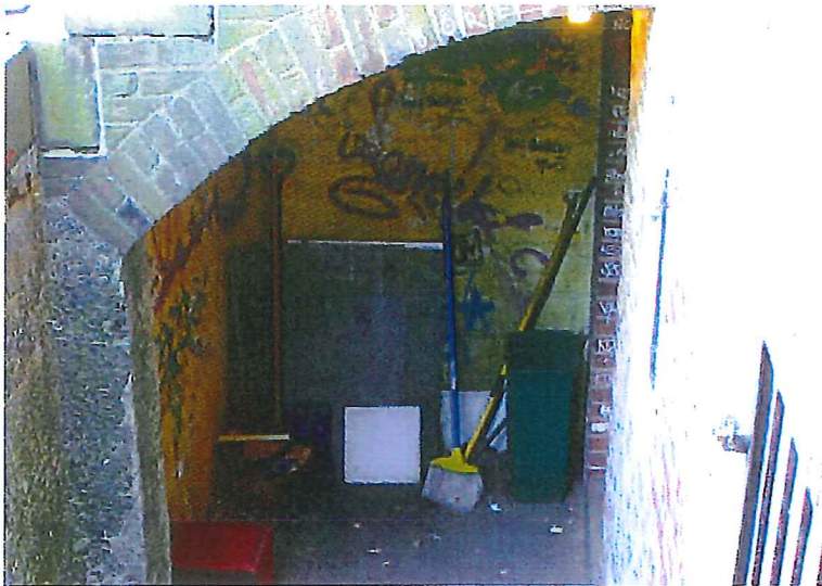
General conditions of parging coating under front step arch
