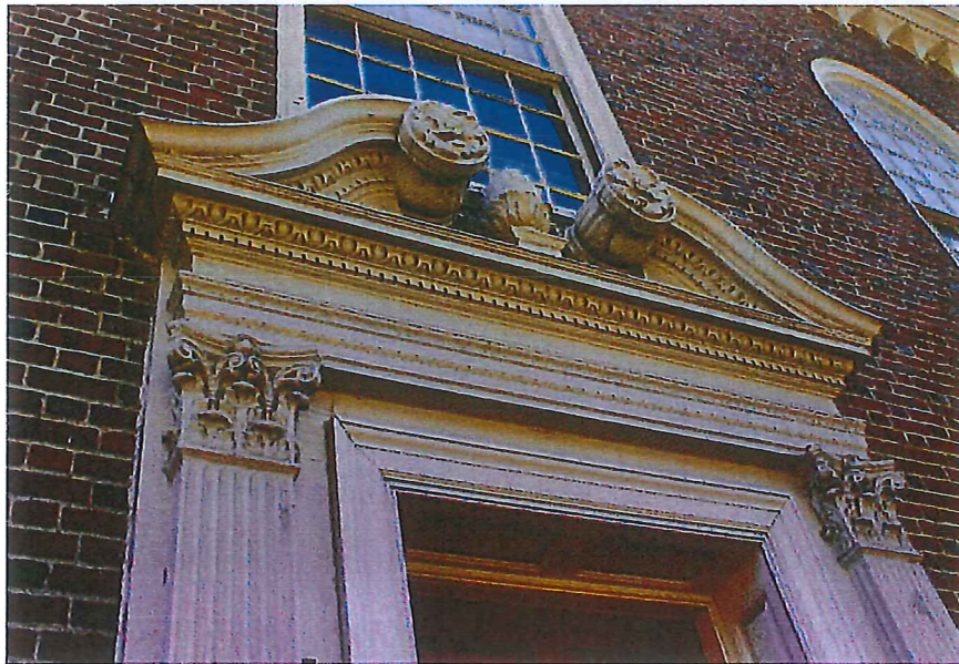
General paint conditions of front entrance surround
