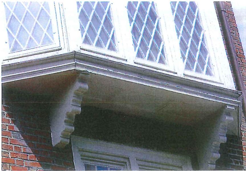
General paint conditions at rear elevation bay window structure
