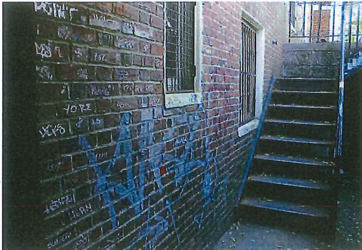
Graffiti visible on walls of front elevation below grade
