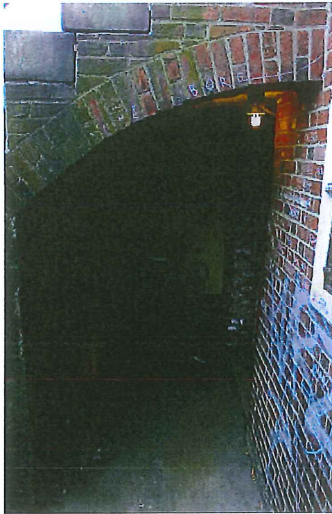
Archway under primary entrance steps Door is located to the right, under the archway
