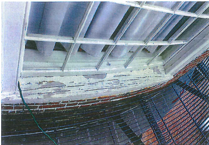
General conditions of wood window sills
