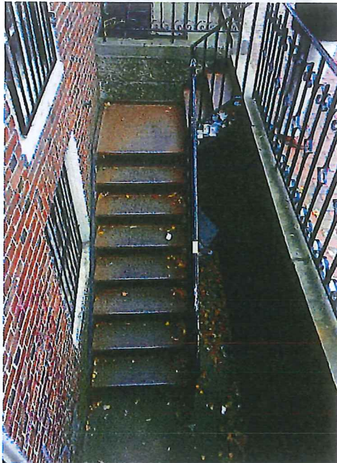
Existing stairway to basement entrance. Existing non-compliant handrail to remain. New compliant handrail to be installed and run along wall.
