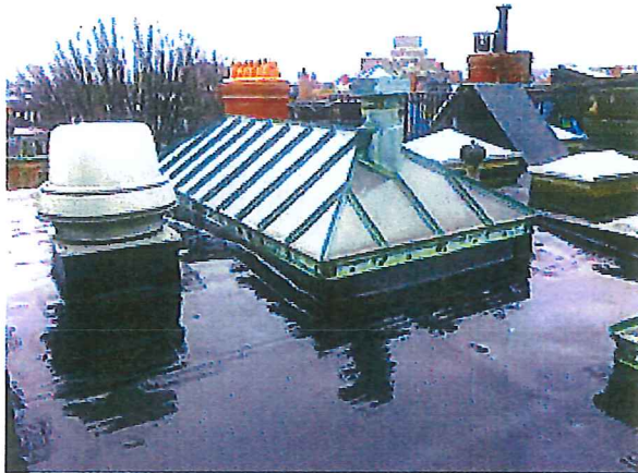
Skylight of the College Club, 44 Commonwealth Avenue, Boston This skylight appears to be similar to that originally drawn for 72 Mount Auburn
