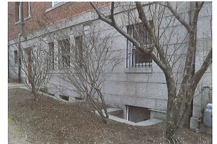
AREAWAY WITH WINDOW TO BE REMOVED
