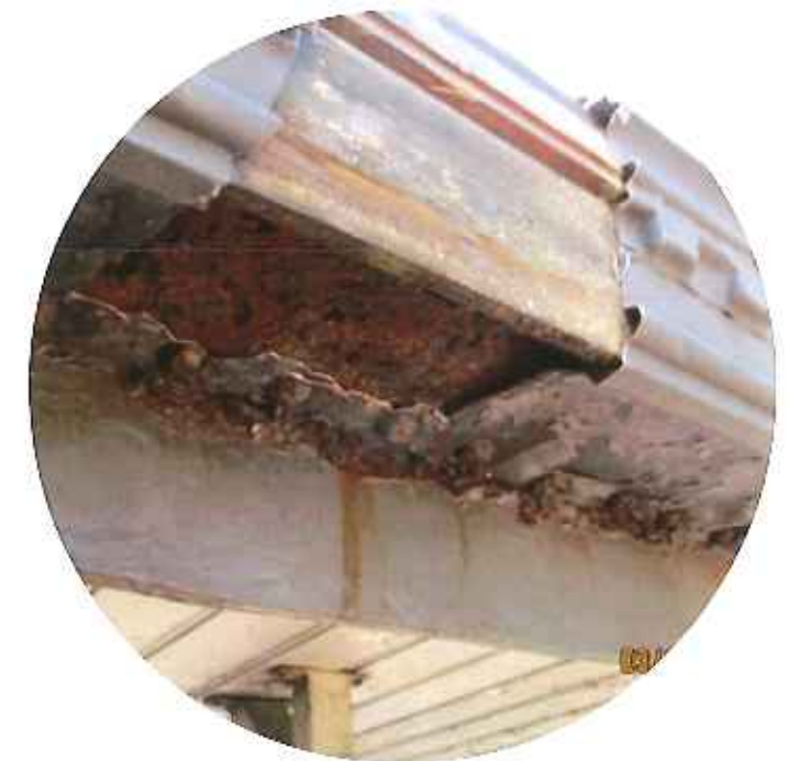
oxidization of the horizontal leg of the steel cornice angle significant oxidization due to a dissimilar metals reaction and water infiltration
