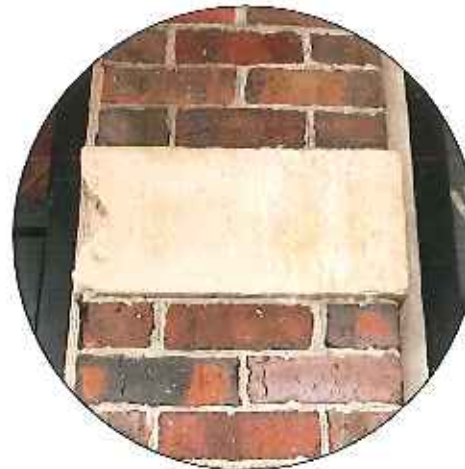
2 limestone spall / dutchman
