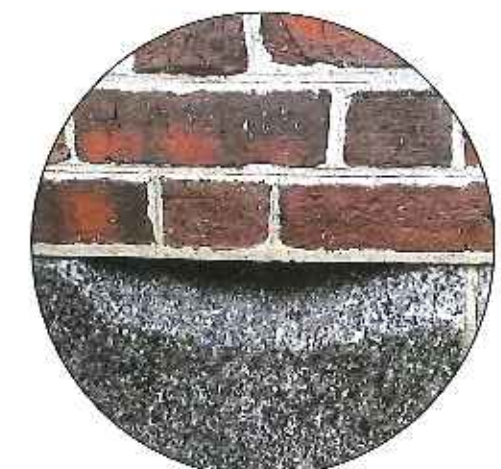
8 granite spall / dutchman
