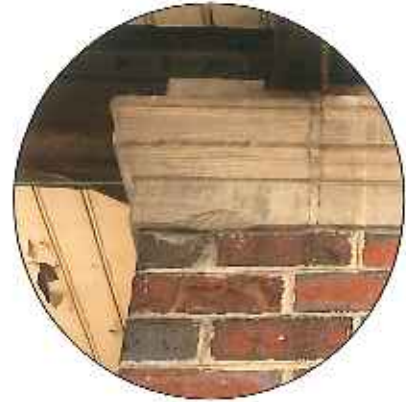
1 spall / no repair
