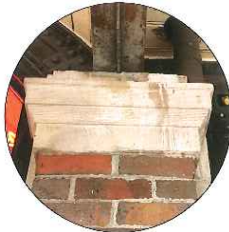
1 limestone spall / dutchman
