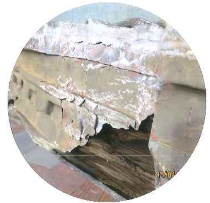
replacement of perimeter dentilled fascia to 1927 details existing lead coated copper to be replaced with new red copper and let to weather
