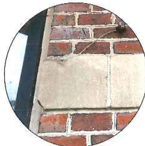
5 two small spalls / one dutchman at end of stone
