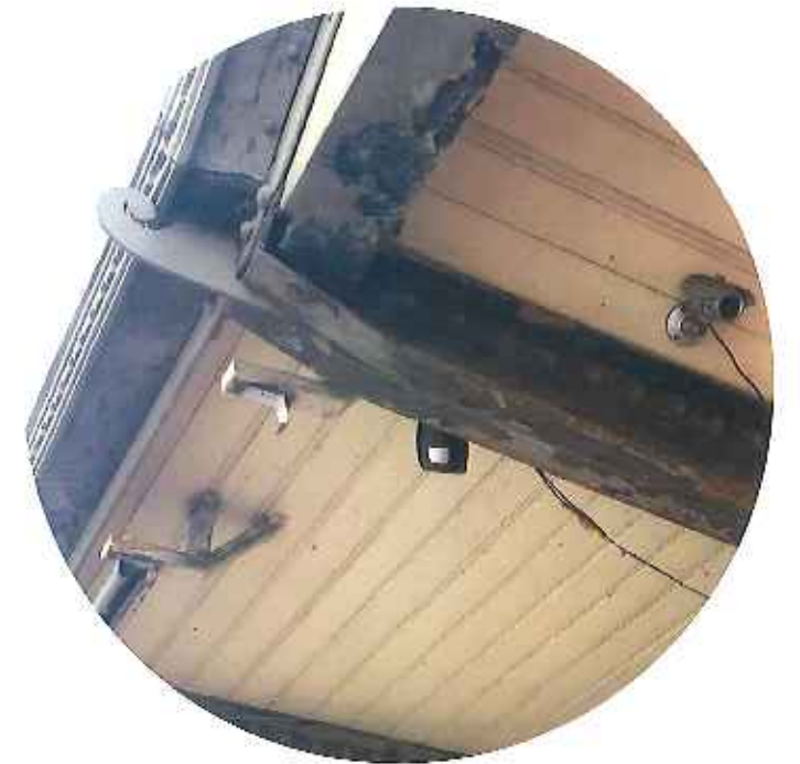
clean structural members for removal of rust and paint, to be repainted in the historic color
