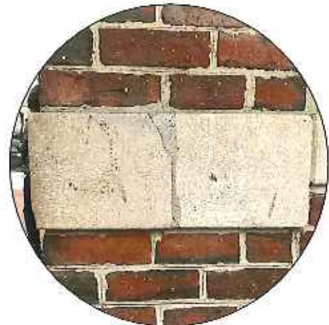
3 limestone spall / dutchman
