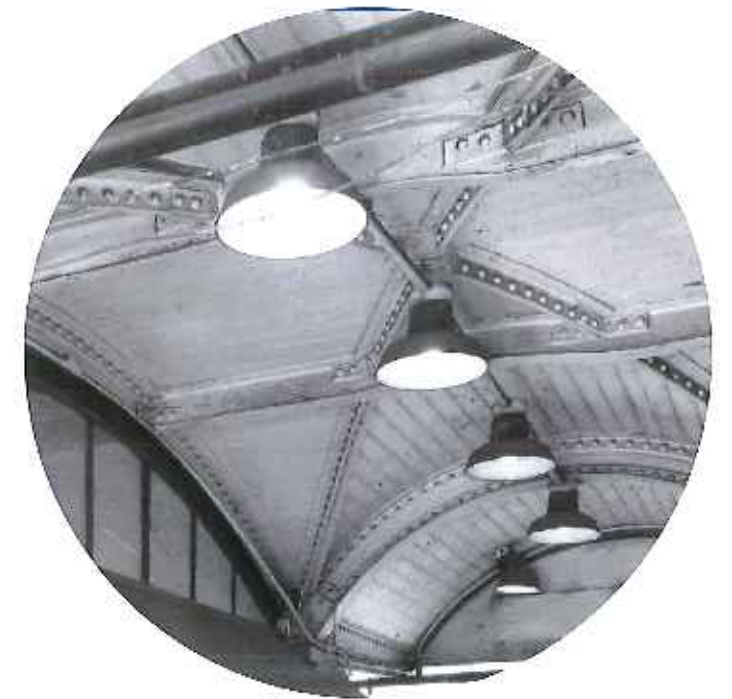
1977 RLMs surface mounted to junction box
