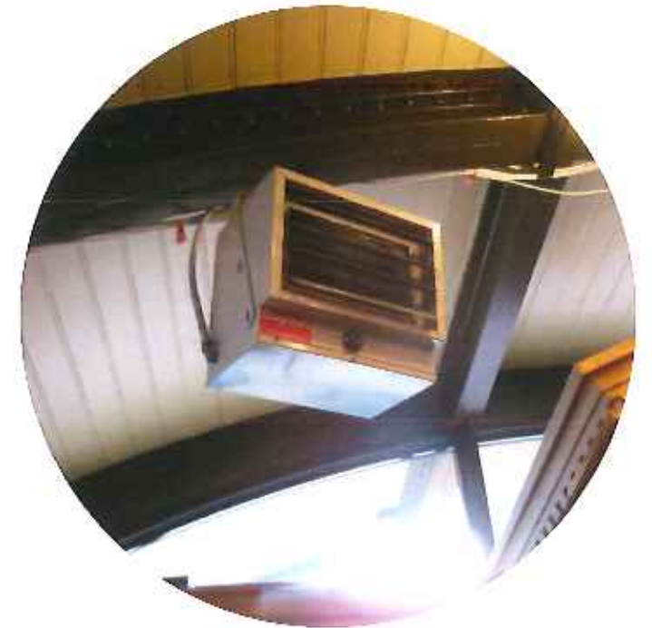
removal of all interior & exterior heating and cooling units for redesign of systems for greater efficiency
