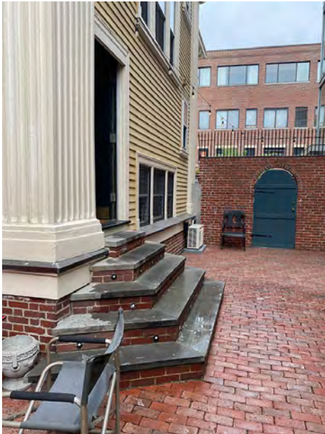
Detail at Courtyard and Stairs to Back Door with Driveway Wall Beyond to North
