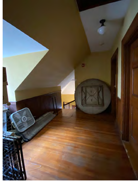
Third Floor Hallway Looking South Toward Back Stair with Headroom 47" at Left and 76" at Right Side of Path to the Back Stairway Due to Roof Slope
