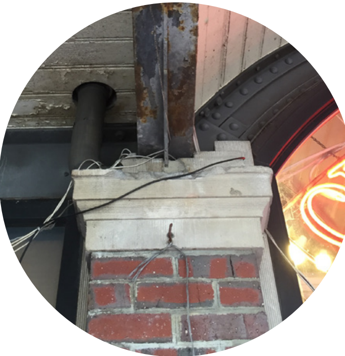
repointing of mortar joints to maintain color, texture and profile of original joints
