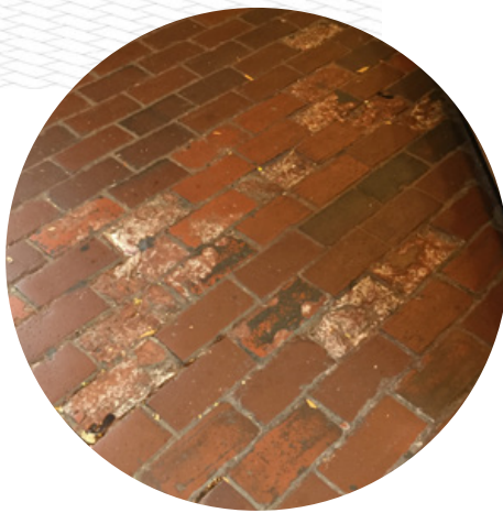
address MAAB compliant brick floor
