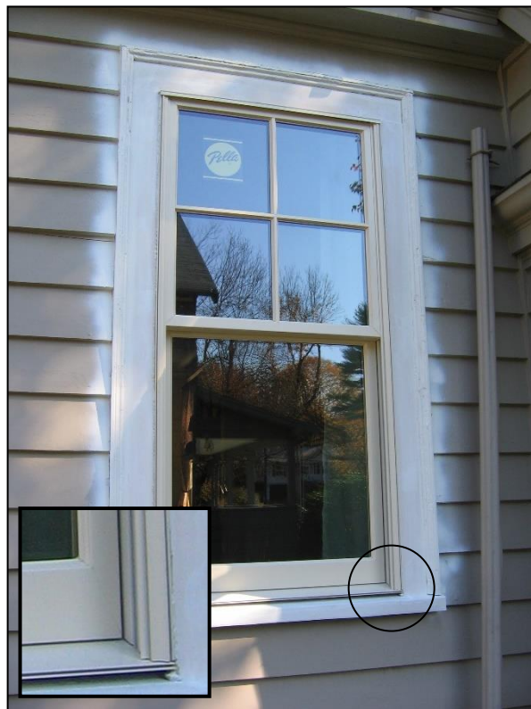
Figure 6: An example of a window insert replacement (note the reduction of the window's rough opening due to the additional framing required to hold the sash)
