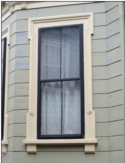
Figure 5: A restored double-hung wood window with a new storm window helps maintain the historic character of a building
