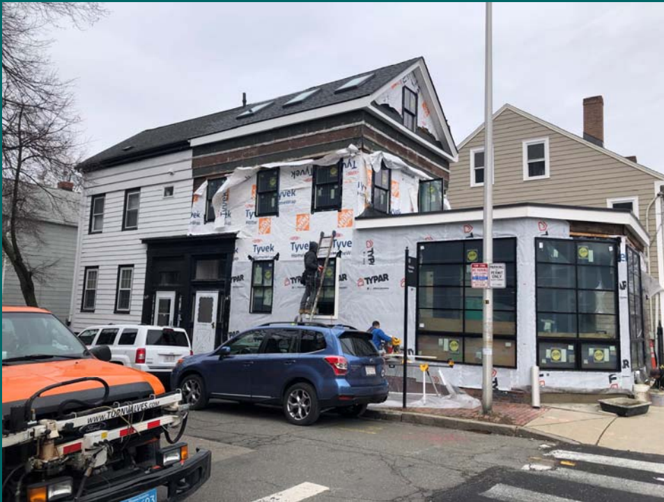
147 Otis Street, later commercial addition being converted to additional square footage for new family.
