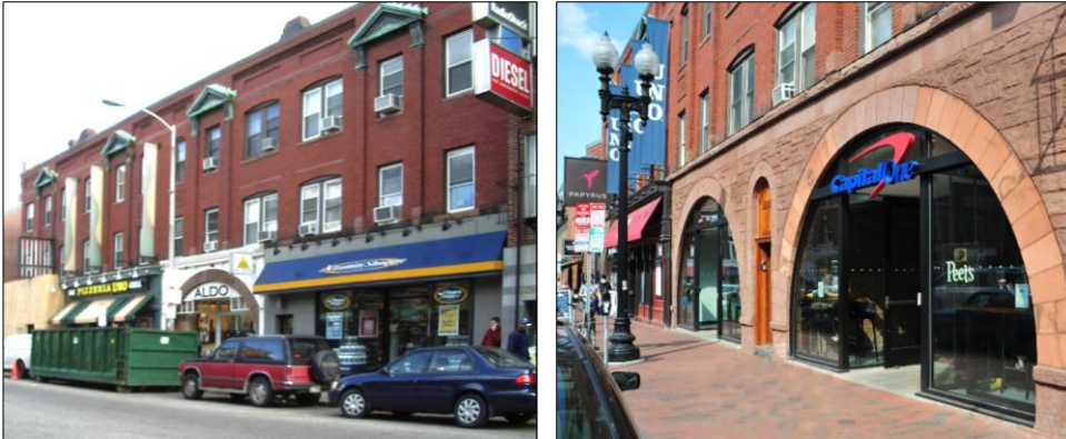
Read Building, 18-28 JFK Street, before and after arch restoration; Cases 1599 (2004) and 3439 (2015). CHC photos.
