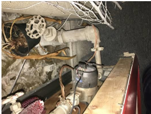
Domestic Water Service & Meter
