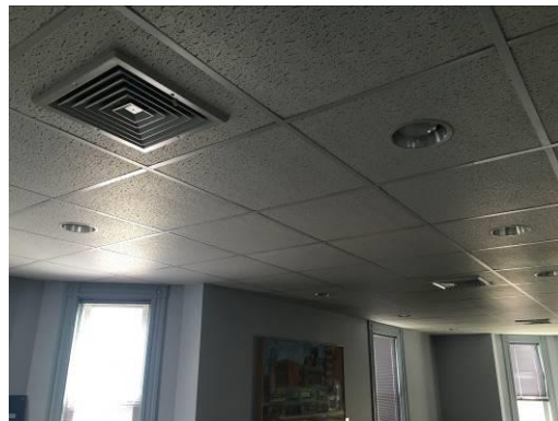
Chamber Room Lighting
