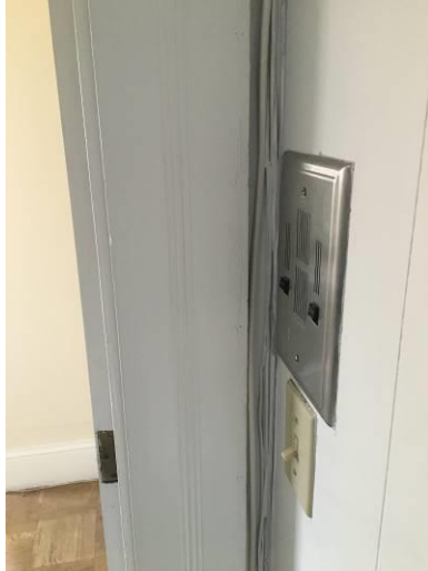
Control Panel & Keypad
