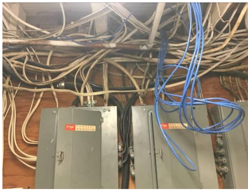
Typical Romex Wiring
