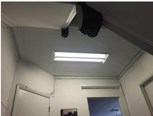
Typical Surface Fixtures
