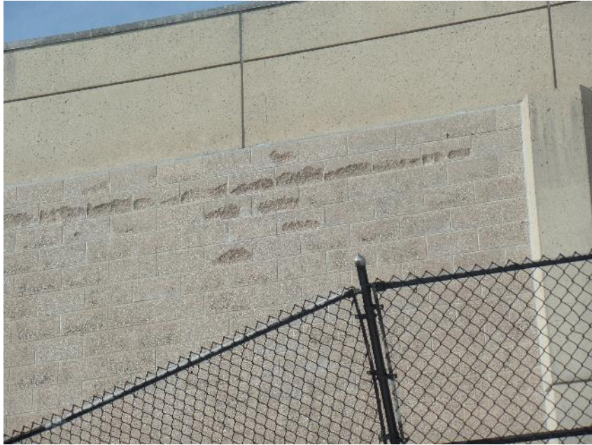
Photo 15: Exterior Masonry Wall - Surficial Damage
