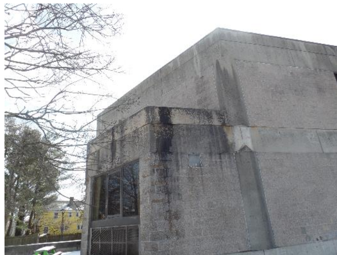
Photo 12: Exterior Masonry Wall -Moisture Damage
