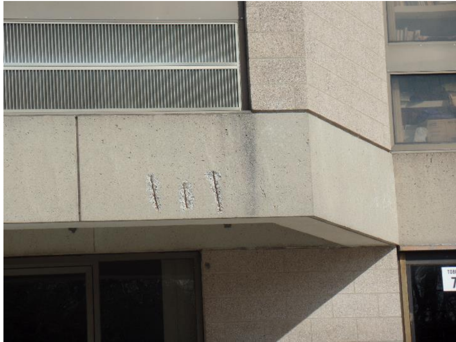
Photo 3: Corroded Reinforcing/Spalled Concrete Cover
