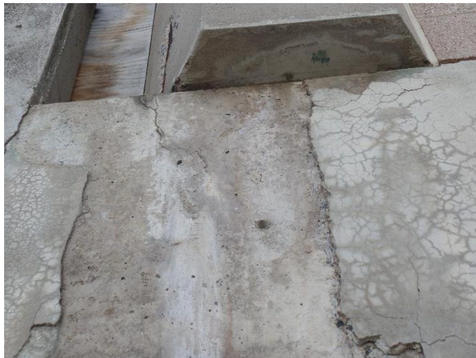
Photo 4: Corroded Reinforcing/Spalled Concrete Cover and Surface Deterioration
