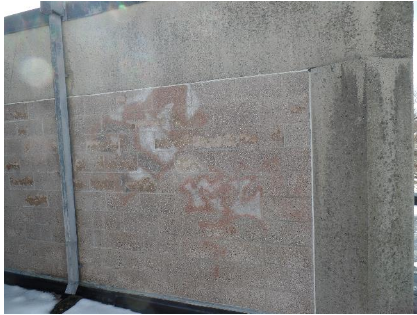
Photo 9: Exterior Masonry Wall - Moisture Damage
