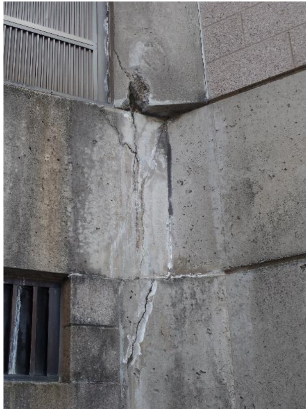
Photo 7: Corrosion/Spalled Concrete Cover and Cracking/Deterioration
