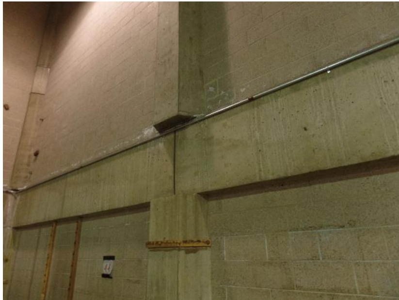
Photo10: Efflorescence on Interior Face of Exterior Wall
