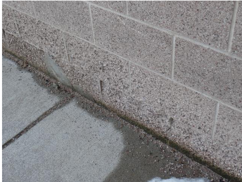
Photo 13: Exterior Masonry Wall - Surficial Damage at Walkway
