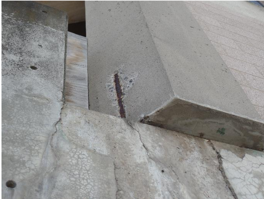
Photo 5: Corroded Reinforcing/Spalled Concrete Cover
