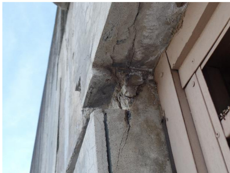
Photo 8: Corrosion/Spalled Concrete Cover and Cracking/Deterioration
